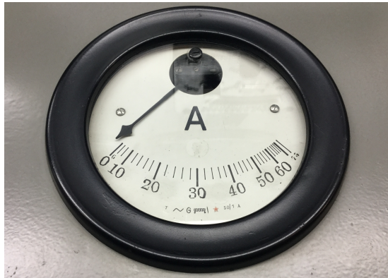
Figure 12.2: Ammeter from the Tagus power plant (currently the Museum of Electricity), Lisbon. Notice that the scale is not linear.
