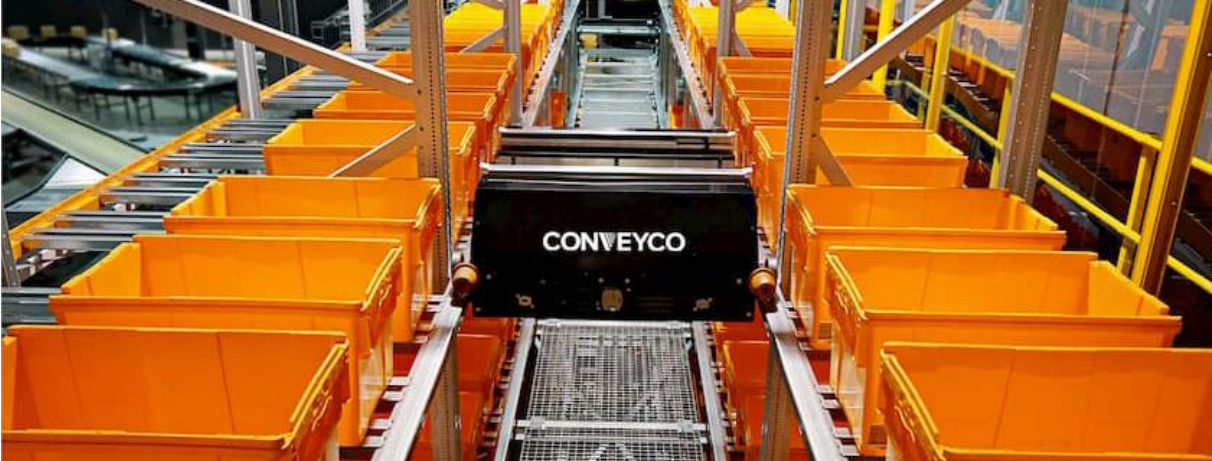
Figure 6 SBS/RS Miniload | Source: https://www.conveyco.com/blog/automated-storage-and-retrieval-types/
