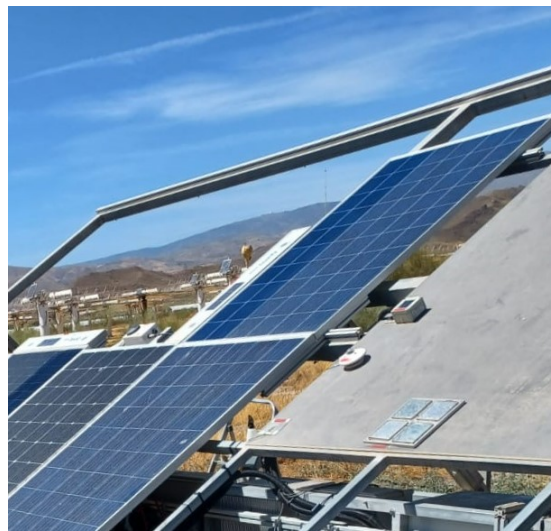
Figure 5.11: Module 1, one substring cleaned. Electrical miss match experience, September 8 th .
