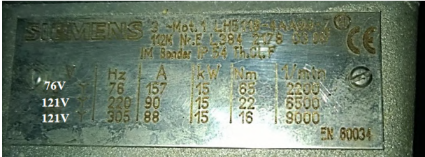
Figure 2.14: Nameplate data of the Induction Motor.
