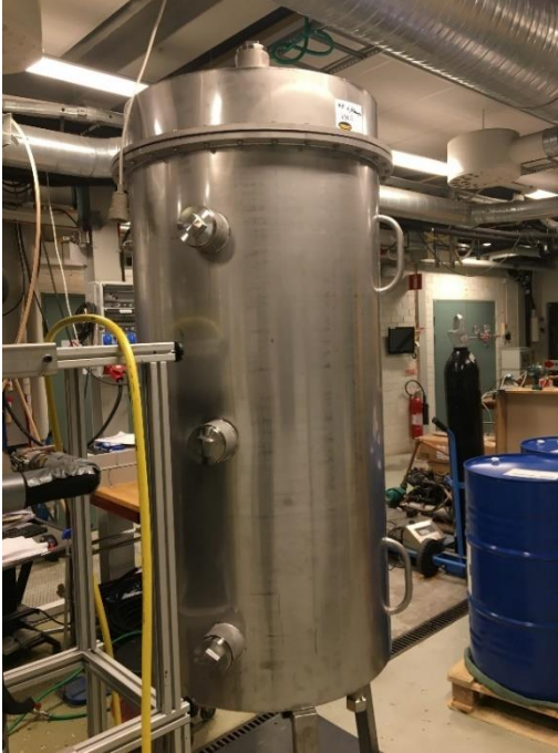
(a) Storage Tank
