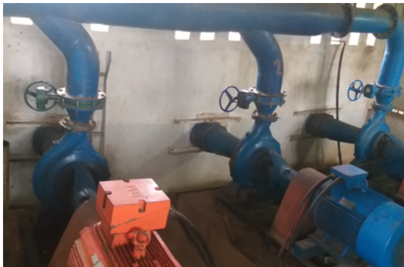
Figure 3.10: Installed pump and motor units.
