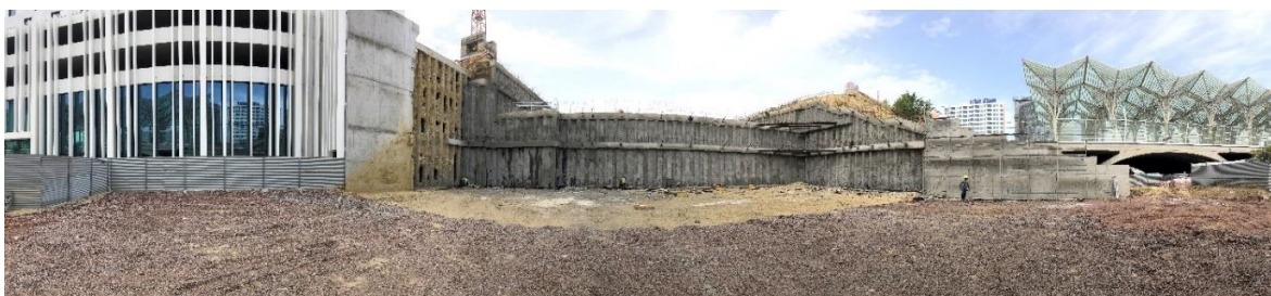
Figure 2 – Anchored spaced pile wall and traditional cantilever wall solution on the South border
