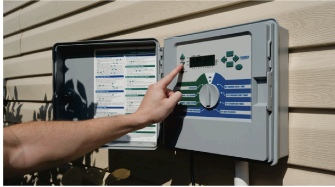
Figure 2-6 Irrigation controller by WaterSense.
