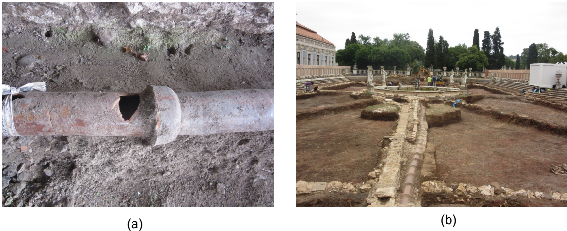
Figure 4-6 (a) Unearthed water pipes from the gardens of the National Palace of Queluz (b) rehabilitation works at Malta garden.
