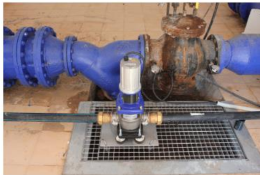
Figure 5.19: Micro-turbine connected to the electric grid with Micro Regen system.
