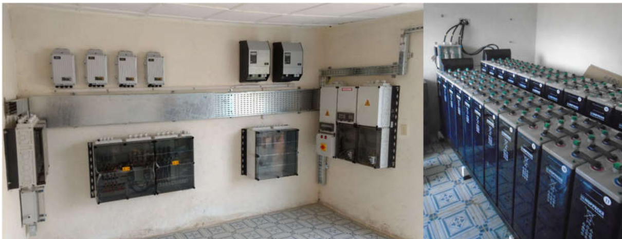
Figure 6.3: Equipment Room (Left) and Battery Bank (Right)
