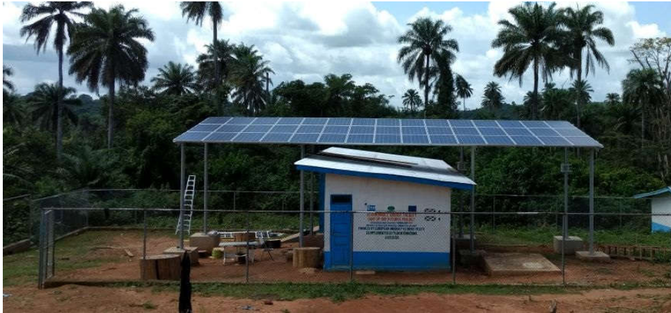
Figure 6.2: Powerhouse and PV Structure
