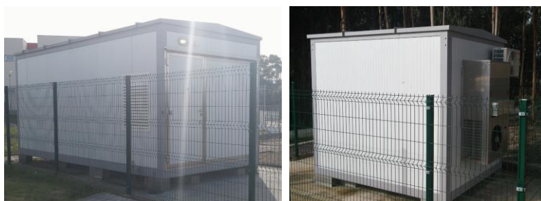
Figure 3-2: Data center geometries: large 20 ft. container (left) and small 10 ft. container (right)
