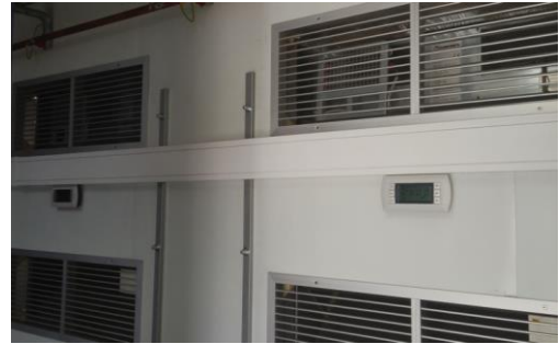
Figure 3-4: Interior supply and return air openings of the PTAC units
