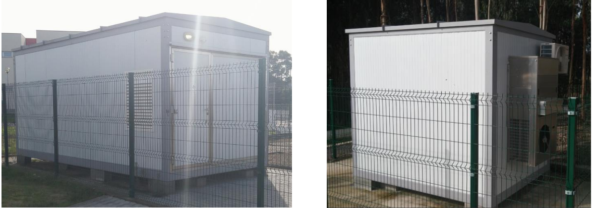
Figure 3-2: Data center geometries: large 20 ft. container (left) and small 10 ft. container (right)
