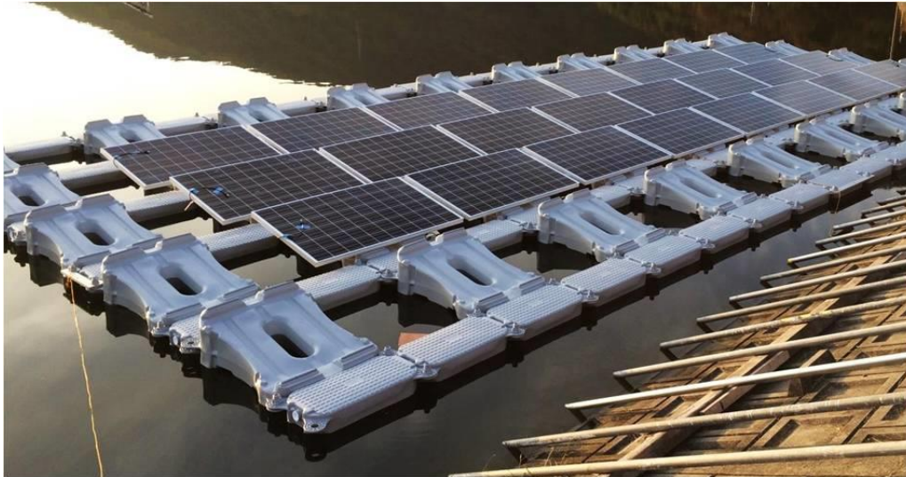
Figure 23: Part of Kagawa's 696 kW plant, installed by Ciel et Terre [38].
