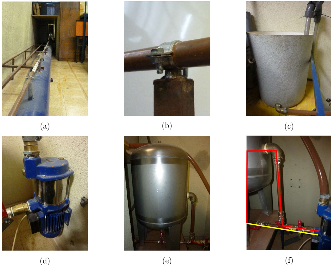
Figure 3.2. Experimental facility components: a) copper pipe; b) pipe metal supports; c) water supply tank; d) pump and needle check valve; e) hydropneumatic vessel; f) operation modes (yellow – derivation; red – by-pass).
