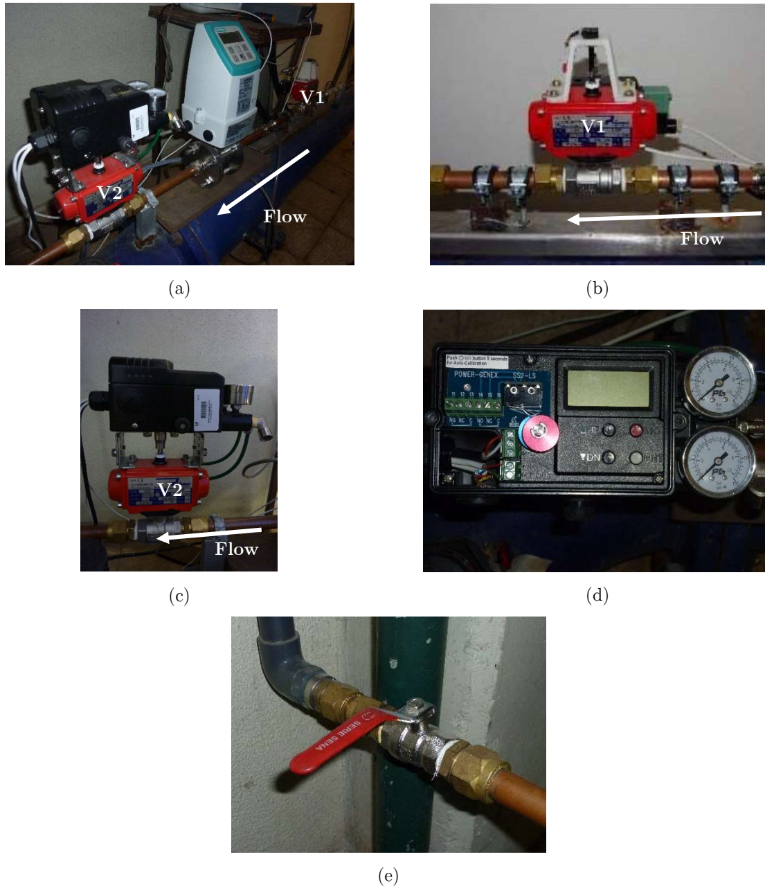
Figure 3.3. Set of valves: a) valve configuration (V1 and V2), b) pneumatically actuated solenoid valve V1, c) position controlled valve V2, d) positioner of the valve, and e) manual flow control spherical valve V3
