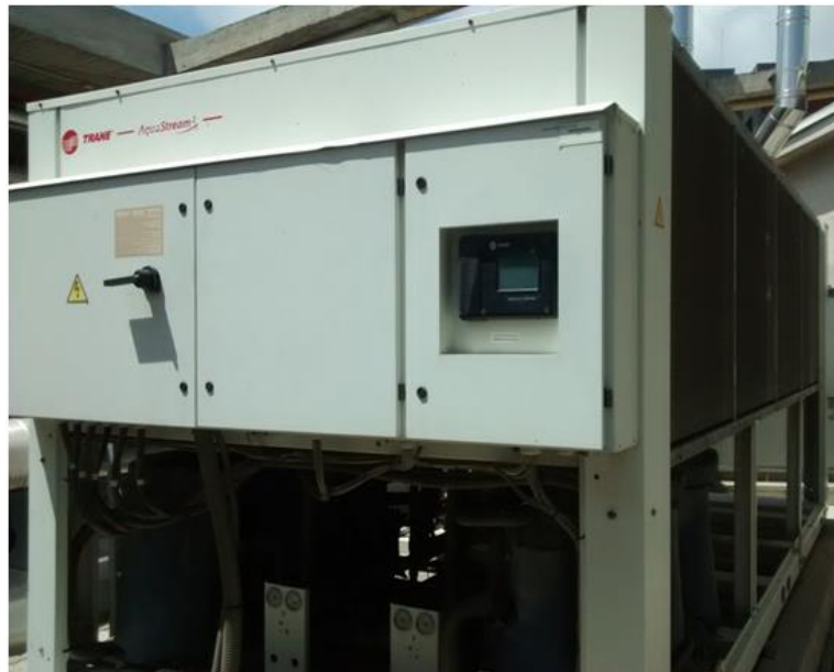
Figure 18 Photo of one of the chillers in ICAEN
