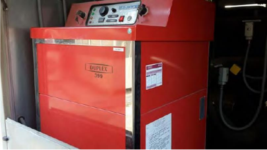
Figure 16 Photo of one of the boilers on the top floor of the ICAEN office
