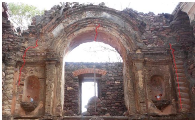
Figure 3 – Cracking and deformation of the altar wall.
