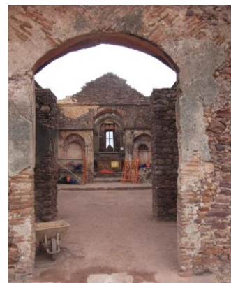
Figure 4 - Disaggregation of masonry.
