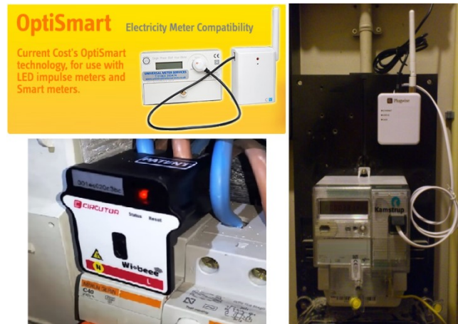
Figure 40. Example of submetering devices (Companies: CurrentCost , Plugwise and Circutor )
