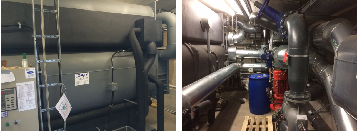
Figure 5.5: Housing of the absorption chiller and its peripheral equipment
