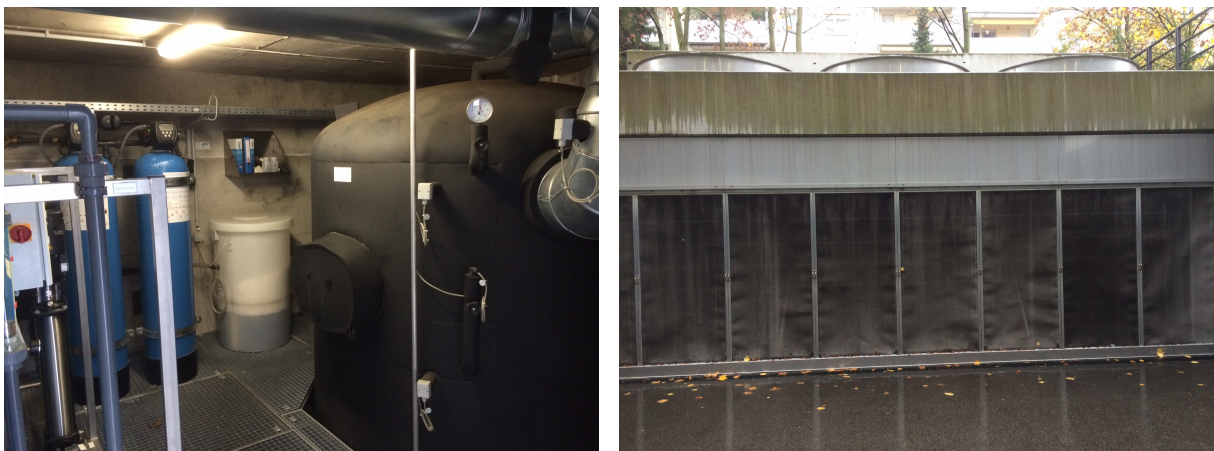
Figure 5.6: Housing of the cold water storage, the water treatment facilities (left) and the hybrid heat rejection system (right)
