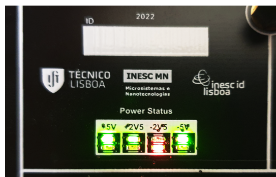
Figure 4.32: Power supervisors LED display with -2.5\text{ V} rail under threshold voltage.
