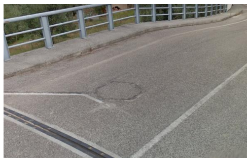
Figure 4.5- Sensors' trigger on the deck of the Várzeas bridge
