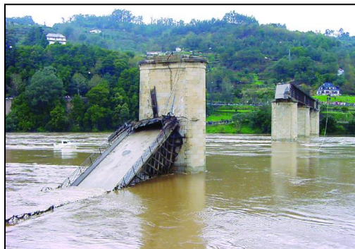
Figure 1.2- Aftermath of the Hintze Ribeiro bridge collapse
