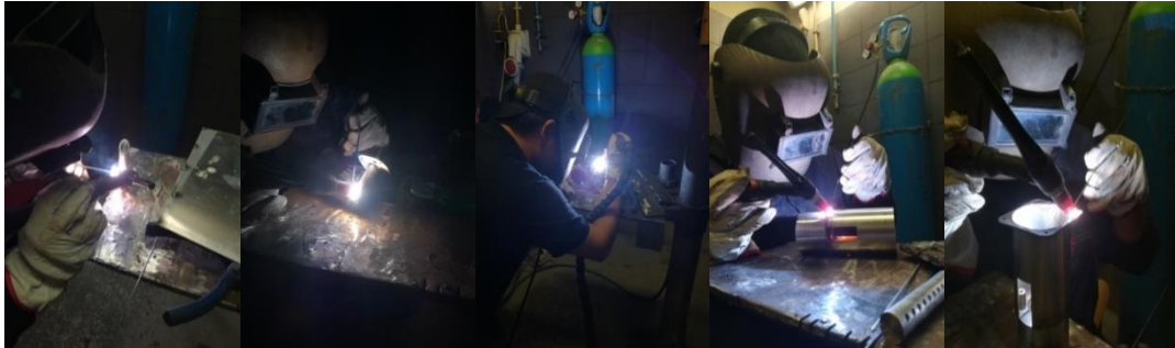
Fig. 41 - From left to right: welding of the handle base; welding of the handle rods; welding of the casing middle; welding of the cup top; welding of the cup base.
