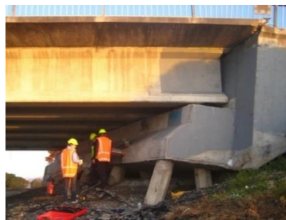
Figura 2.5. Rotura num encontro em Christchurch, New Zealand (2010), [http://www.calit2.net/newsroom/release.php?id=1890]
