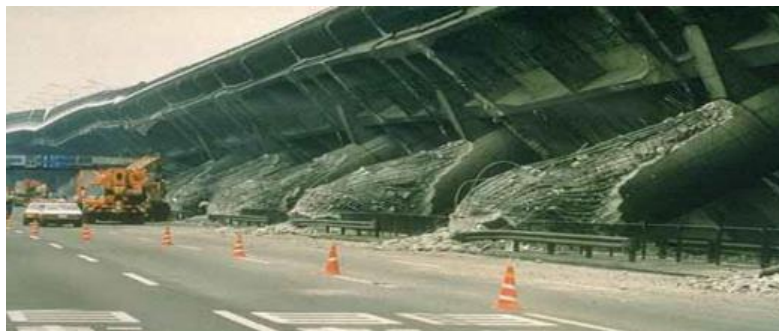
Figura 2.3. Roturas devida a dispensa prematura de armadura longitudinal em Kobe (1995), [https://www.researchgate.net/figure/Flexural-failure-at-the-base-of-bridge-pier-during-1995-kobe-earthquake-Hanshin_fig2_273573779]
