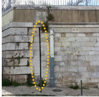
Figure 4 - Fissure in lower retaining wall
