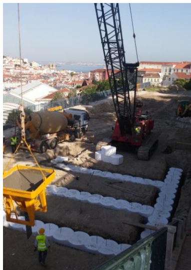
Figure 28 - Stabilization solution: Pile grid location in lower platform; beginning of excavation process
