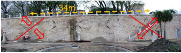
Figure 2 - Cracks in upper retaining wall ( R_{sup} )
