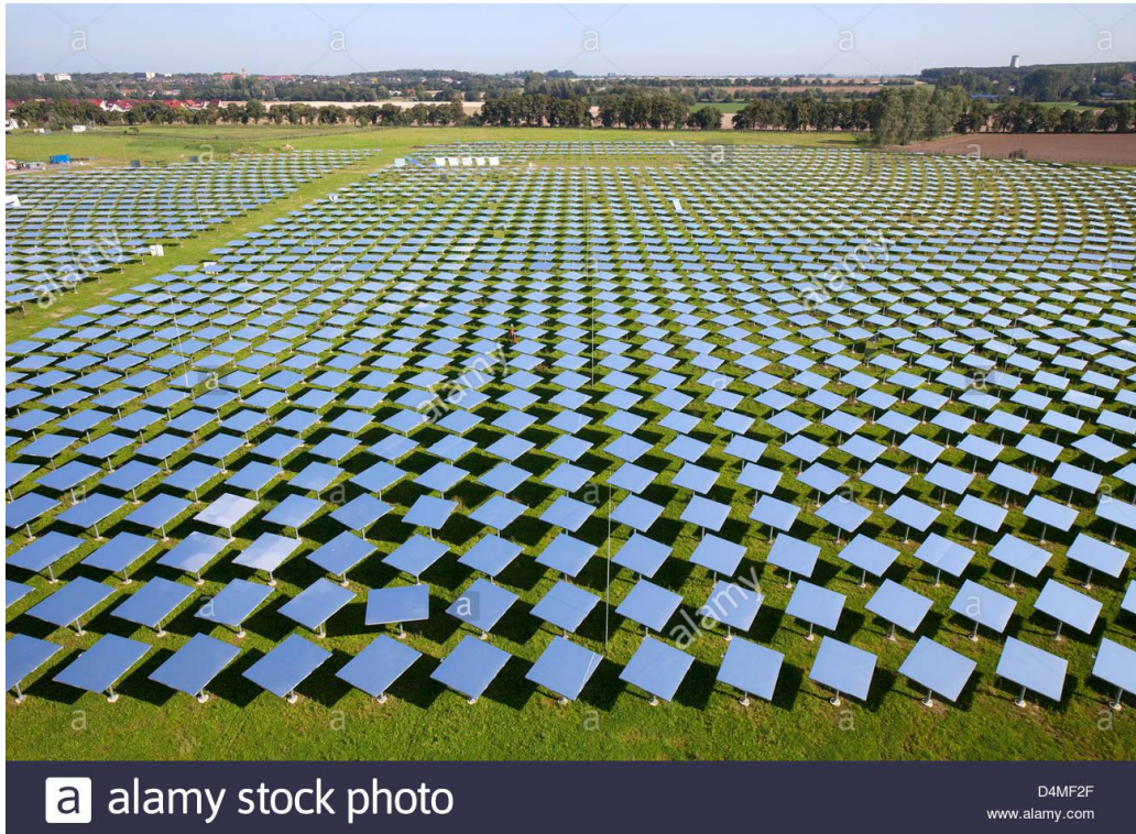
Figure 6-4: Heliostats filed in a solar tower power plant; Source: https://www.alamy.com/stock-photo-juelich-germany-solar-power-tower-juelich-54540599.html .
