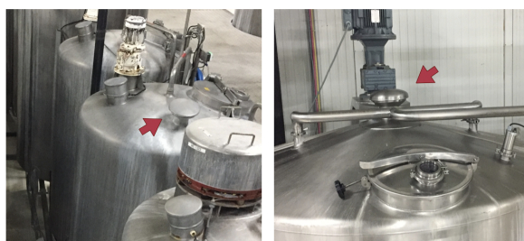
Figure 3.4: Placement of vents in ageing tanks: Old model (left, original photo), New model (right, original photo)
