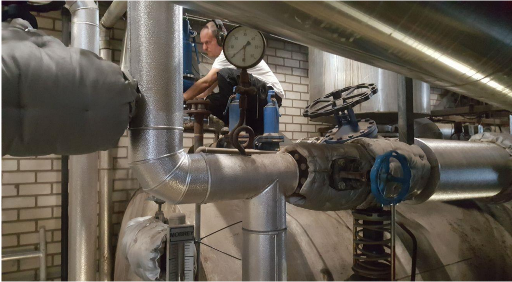
Figure 46 The connection of RCG add-on to the main steam line
