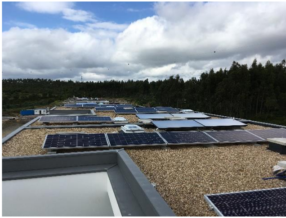
Figure 7 Townhouse 307 renewable energy installation
