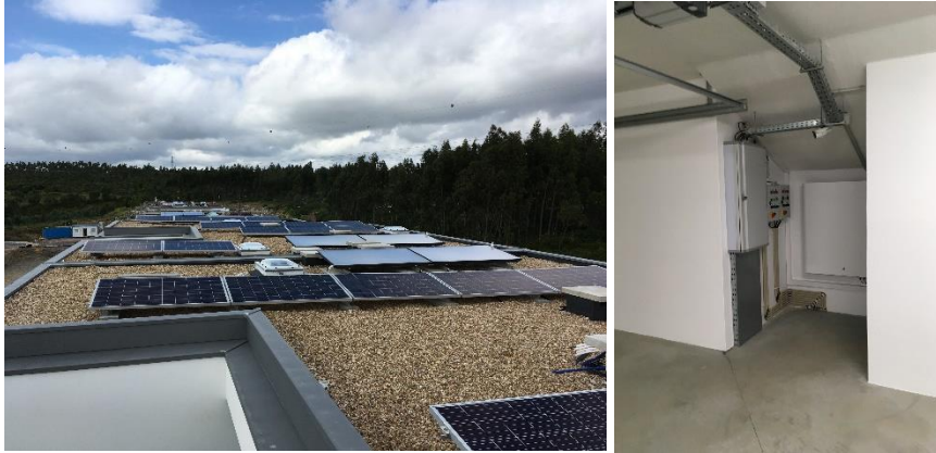
Figure 28 Townhouse 307 solar photovoltaic and solar panel (left) and battery storage (right)
