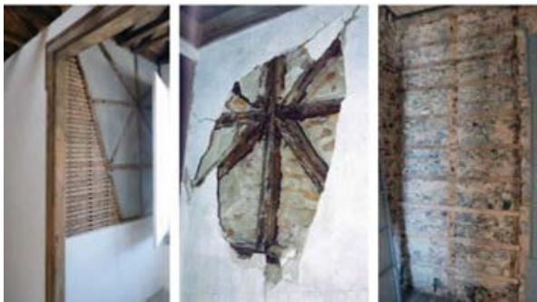
Figure 2-24 – Timber frame partition walls Alfândega building with different geometries (Picture from H.Ea.R.T 2015 [25])
