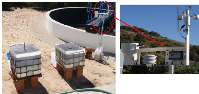
Figure 1 - Pilot installation in the Póvoa da Galega wastewater treatment plant
