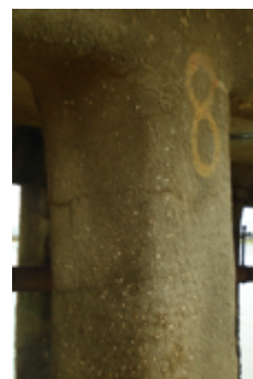
Figure 4 – Transversal cracking – Level B
