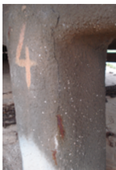
Figure 3 – Longitudinal cracking and rust stains – Level A
