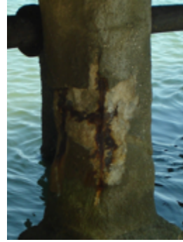
Figure 6 – Extense delamination and exposed of reinforcement – Level D
