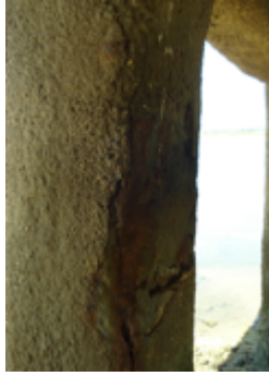
Figure 5 – Extense delamination and rust stains – Leve C
