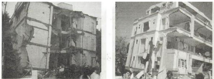
Figure 2.3 – Failure of reinforced concrete buildings with “hanging” columns [1]
